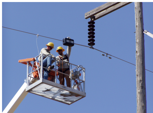
Figure 7: Operation of EMAT System By Linemen
