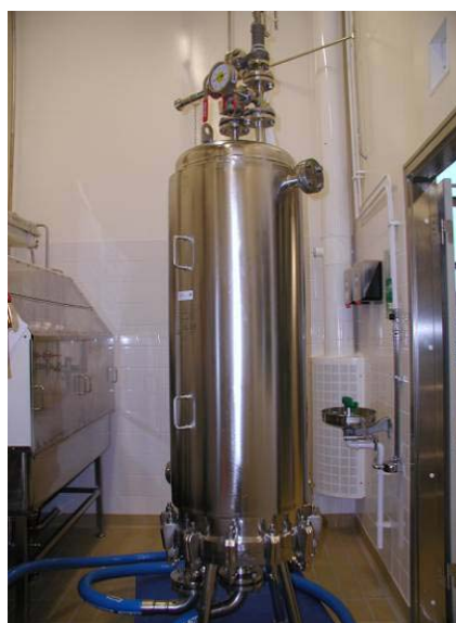
Figure 8: Jacketed PALL filter housing containing four 16” modules
