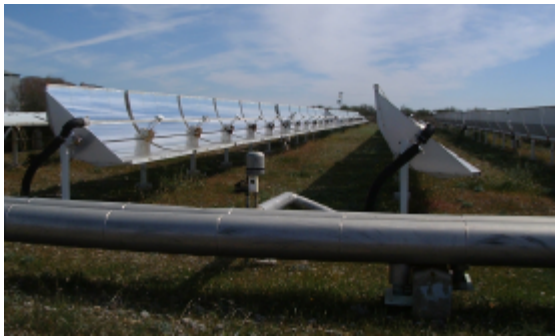
Fig.1 ACUREX Solar collector field.
