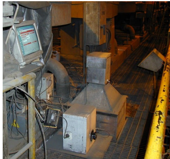
Fig. 2. The actual system running in Pyhäsalmi concentrator
